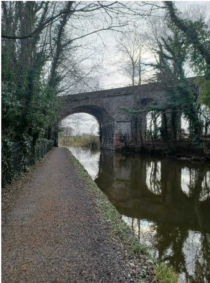
Insert 8.4 - Looking west at the Grade II listed railway viaduct over the Shropshire Union Canal (NHLE 1278977)
